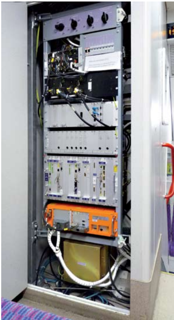
Onboard equipment cabinet of a dual-fitted Class 471 City Elephant EMU, located in the vestibule.
