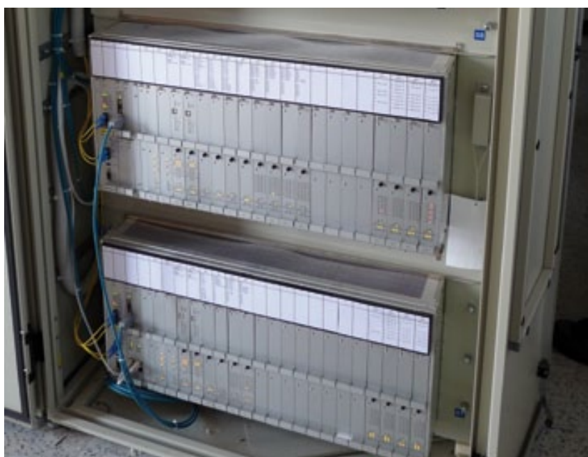
KSZZ modules embedded in EIP panels in railway station Bratkovice
