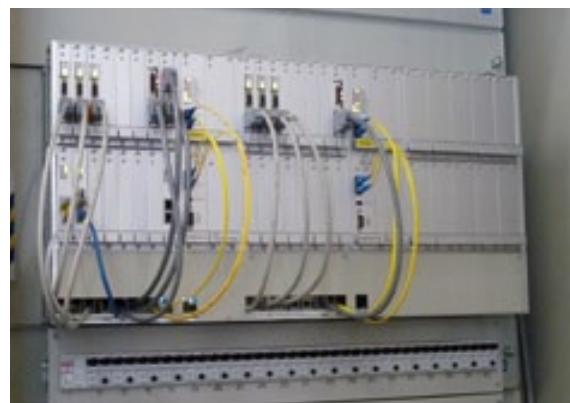
KSZZ panel in ESA 33 interlocking room in railway station Pribram
