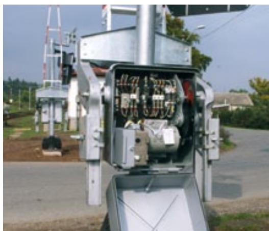
Barrier drive box
