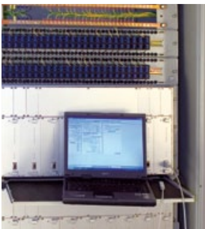
KOA-1 rack with TCR track receivers and diagnostic PC
