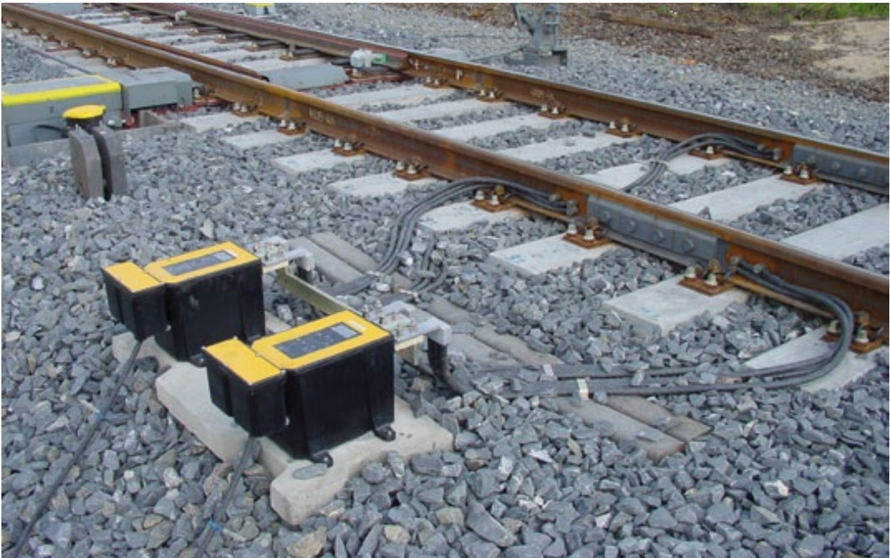
Impedance bonds connected to track circuits
