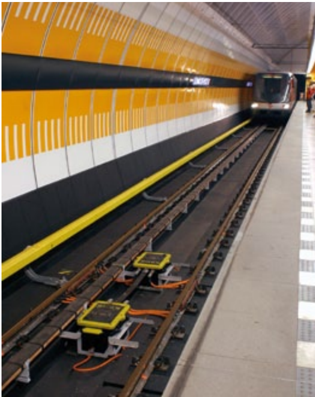
Impedance bonds at metro station railyard
