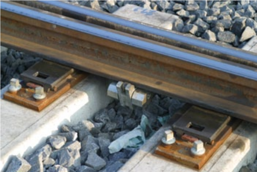
Thrusting roller chair in opened point blade position
