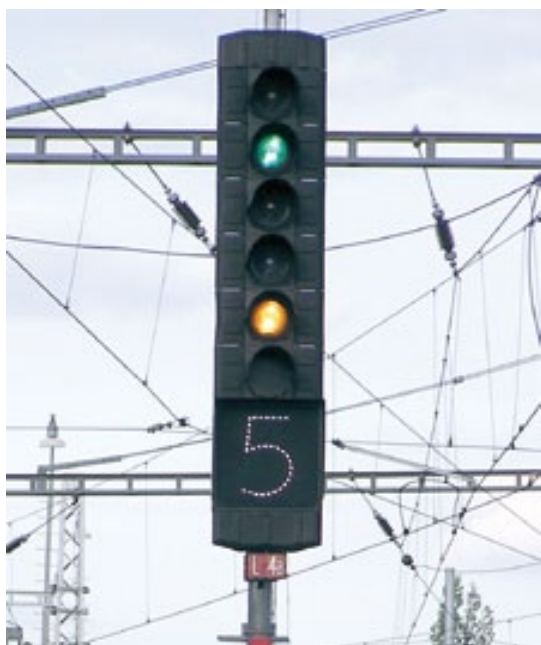
Example of signal lamps set
