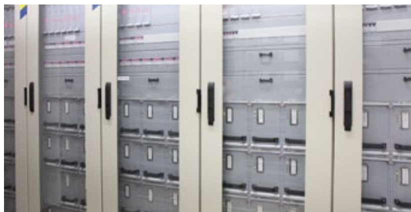
Interlocking room with ESA 11M vital computer cabinets
